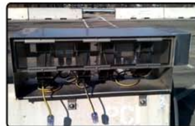
THIS IS ONE OF MANY CHARGING STATION AT CHICAGO TRANSIT'S NORTH YARD PROVIDING RETRACTABLE POWER FOR HUNDREDS OF NEW FLYER ELECTRIC BUSES WHICH ARE USED IN MOST LARGE US CITIES.
