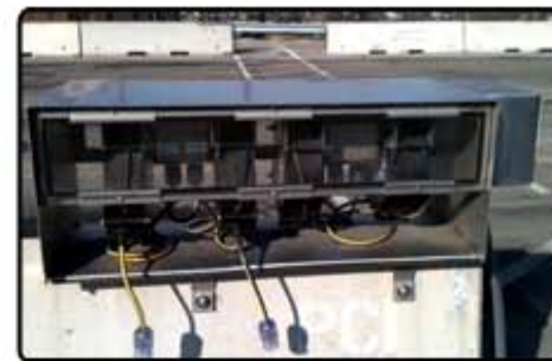
THIS IS ONE OF MANY CHARGING STATION AT CHICAGO TRANSIT'S NORTH YARD PROVIDING RETRACTABLE POWER FOR HUNDREDS OF NEW FLYER ELECTRIC BUSES WHICH ARE USED IN MOST LARGE US CITIES.
