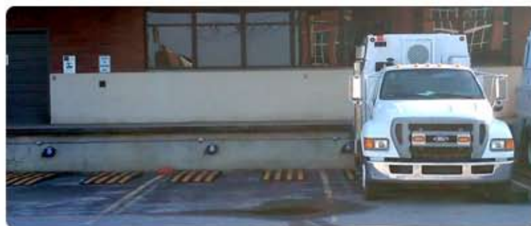
LOADING DOCKS THROUGHOUT NORTH AMERICA HAVE BENEFITED FROM THE ARCTIC LEASH IN HEATING DIESELS, CHARGING REFERS, AND ELIMINATING LOST AND STOLEN CORDS LIKE THIS DELMARVA FACILITY IN NEWARK DELAWARE.
